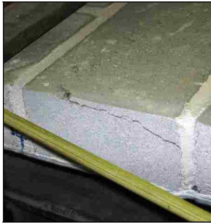
(a) Flexural-Shear Cracking
