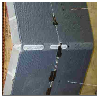
(b) Rupture of Polyurea
