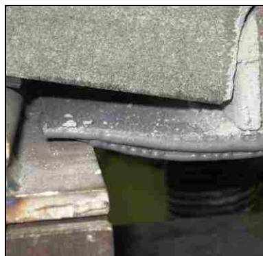
(b) Debonding of Polyurea
