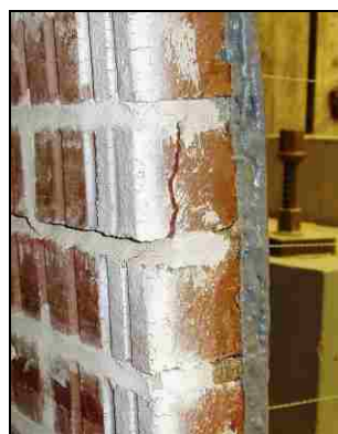
(b) Flexural-Shear Cracks
