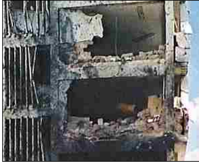
Figure 1.2. Failure of Exterior URM Infill Walls
