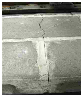
(b) Longitudinal Cracking
