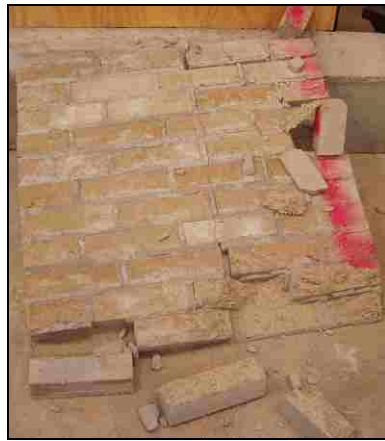
(a) Wall Collapse
