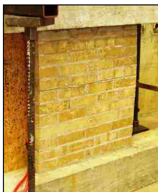
(a) Horizontal Cracking
