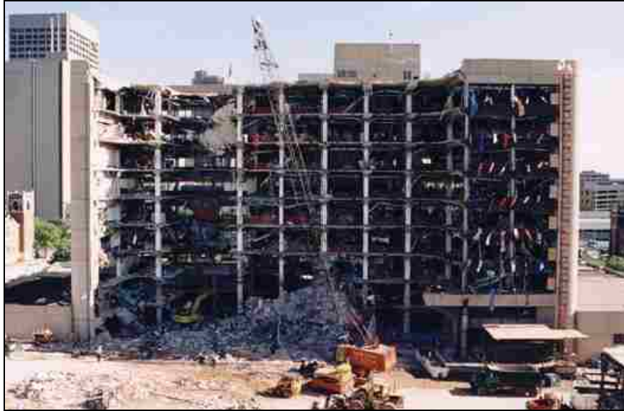
Figure 1.1. Damage to Alfred P. Murrah Building (FEMA, 2003)
