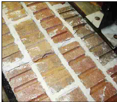
(a) Longitudinal Cracking
